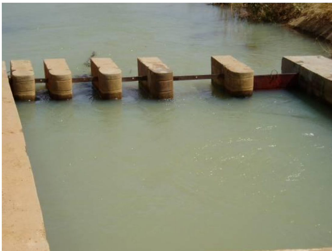
Plate 5: Kadawa Sector Turnout with missing metal shutters
